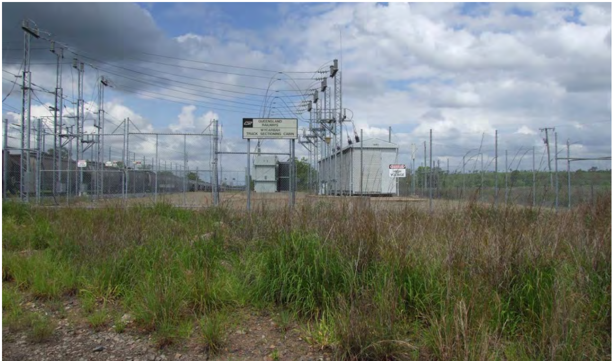
Figure 5: Example of a Track Sectioning Cabin (TSC)
