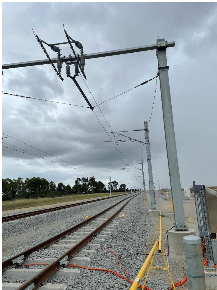
Figure 6-4 60kg/m rail on TAL sleepers and overhead line equipment
