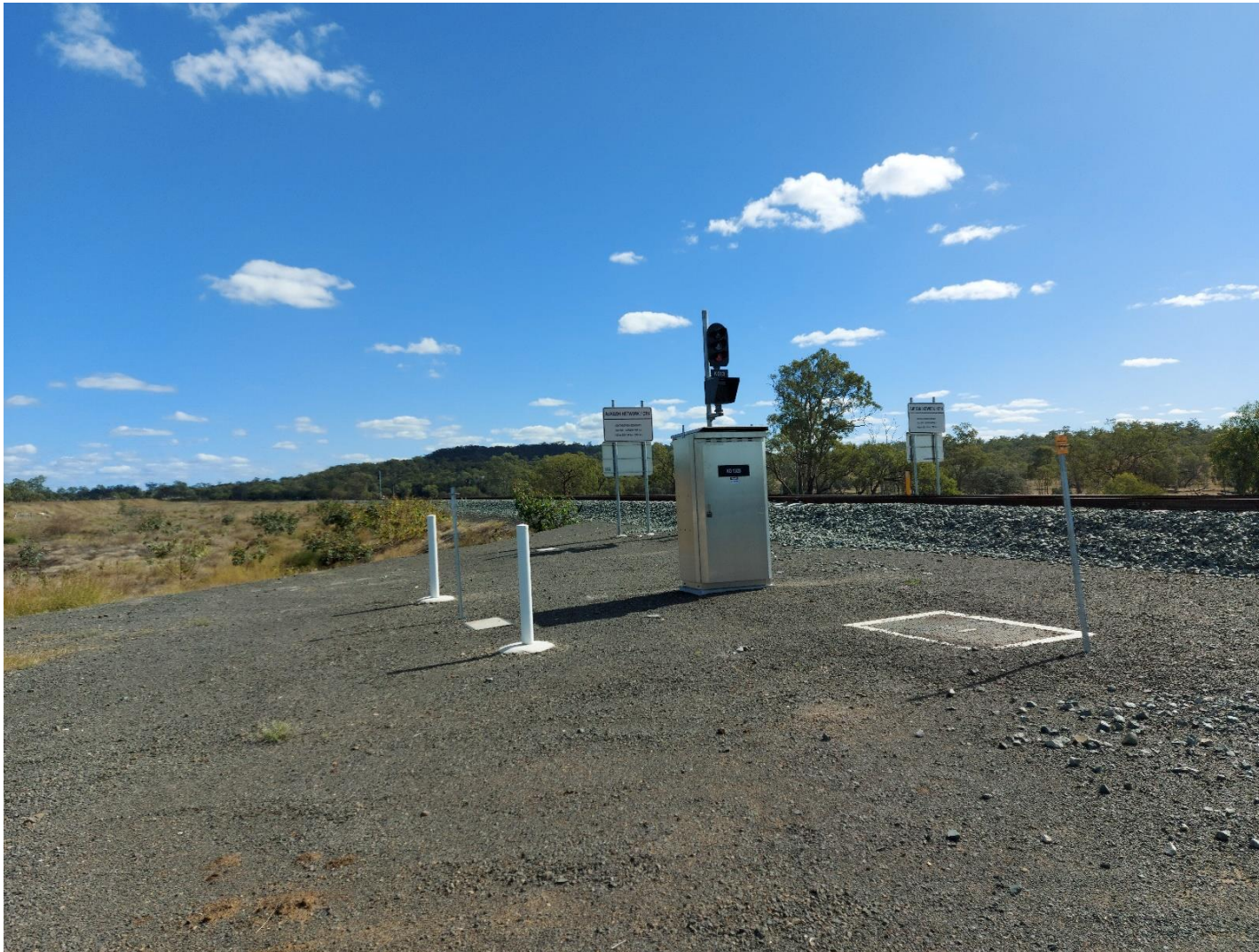
20220726_135551 – Signalling Equipment - Looking West
