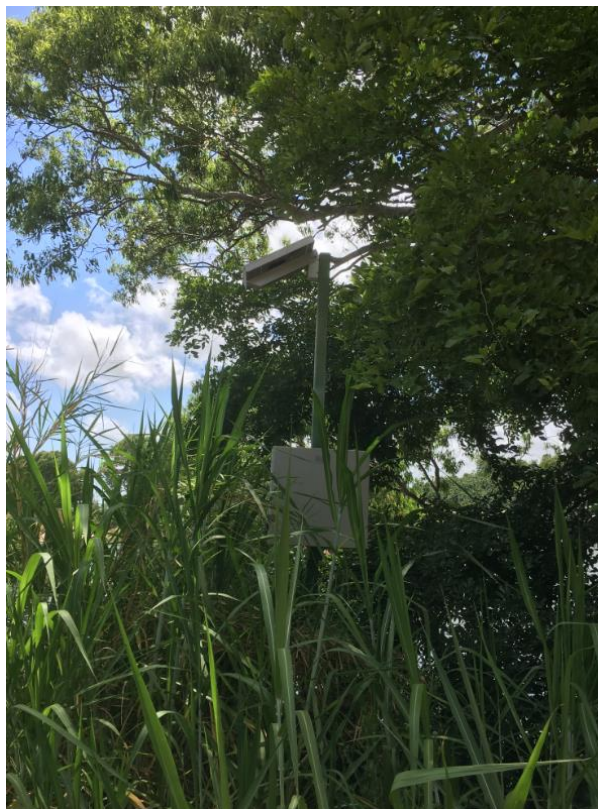
Figure 3-10 – Giru Weir – Level Gauge
