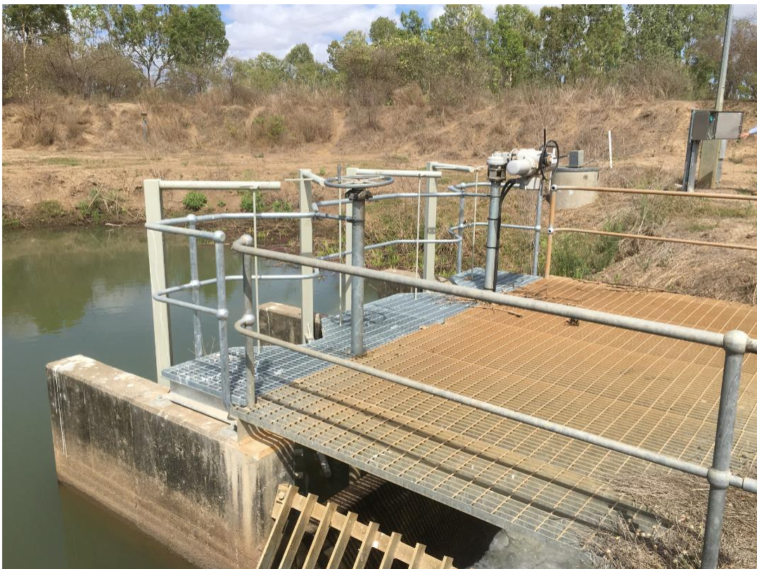
Figure 3-2 – Haughton Balancing Storage – Release Gates to Haughton River
