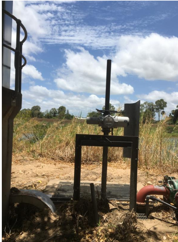
Figure 3-17 – Healeys Lagoon Pump Station on Val Bird Weir
