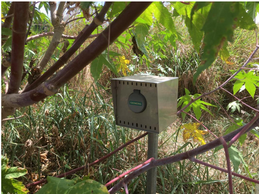
Figure 3-12 – Giru Weir Bypass Pipe Gauge
